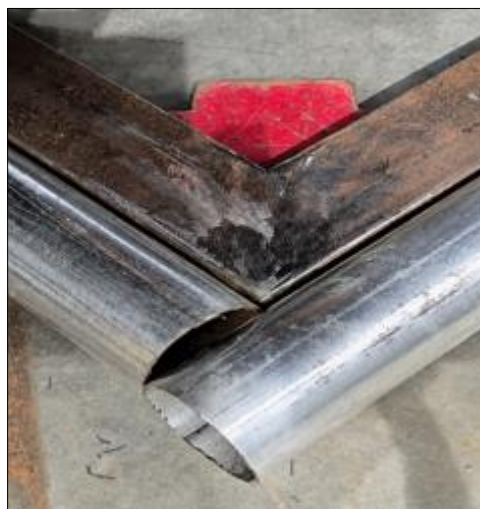
Fig 3: Mitred corner joint of round steel tubing showing an open root gap and a partly cut, unclosed section of the tube wall.
